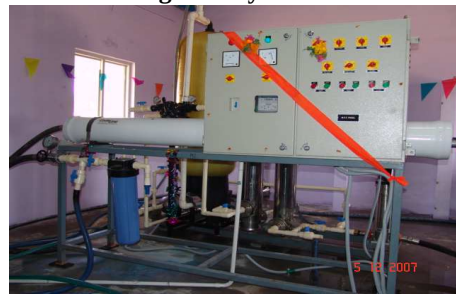
R O Plant (inside view)
